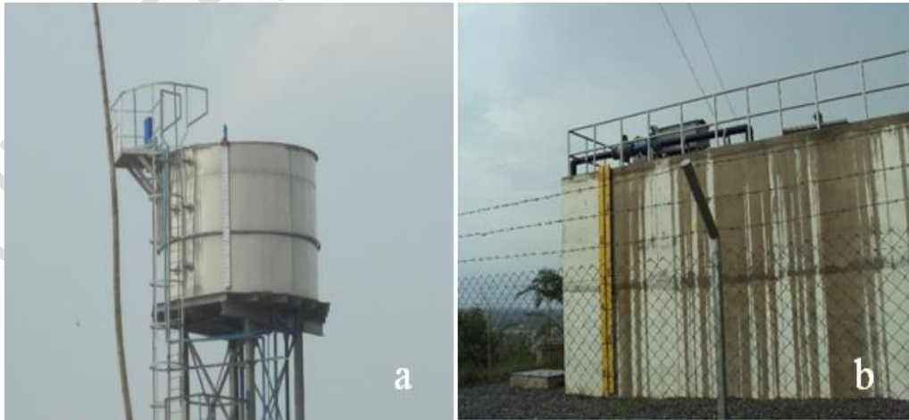
Plate 4. Service reservoirs of the AFSTWSS (a) Elevated aluminium reservoir; (b) Ground-level concrete reservoir (Source: ANMA [20])
