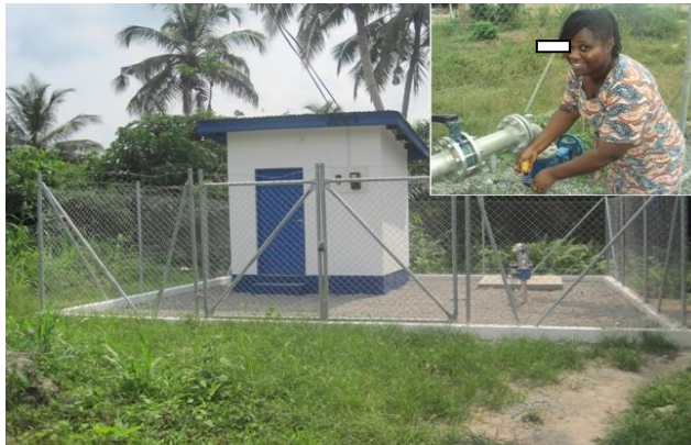
Plate 2 Water source – borehole and pumping station – at Assin Fosu (Credit: Authors)
