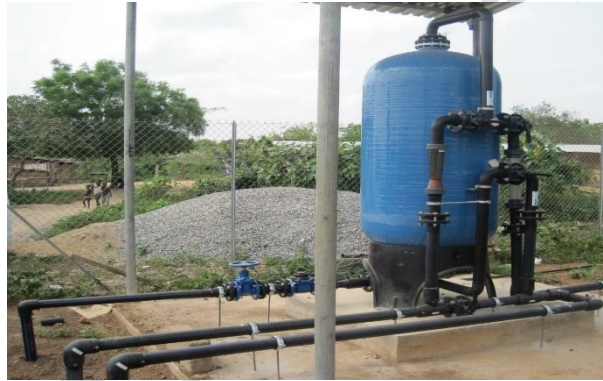
Plate 3 An Aquatec filtration unit installed in the AFSTWSS (Source: ANMA [20])
