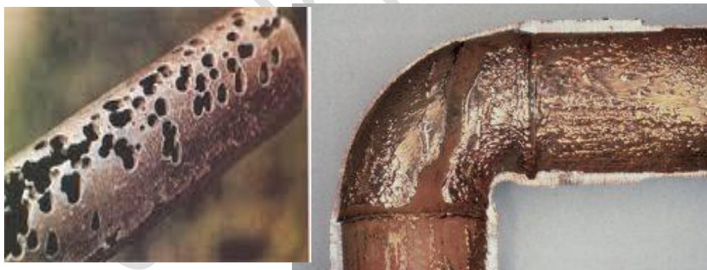
Plate 1. The effect of corrosion on metal pipes
