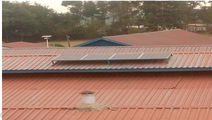
Figure 1: Photograph of the installed PV Array on the institution's social/ dining hall roof.
