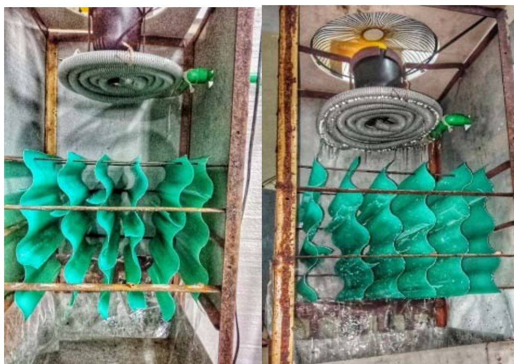
Figure 8. Cooling tower with film fills with ripple plates
